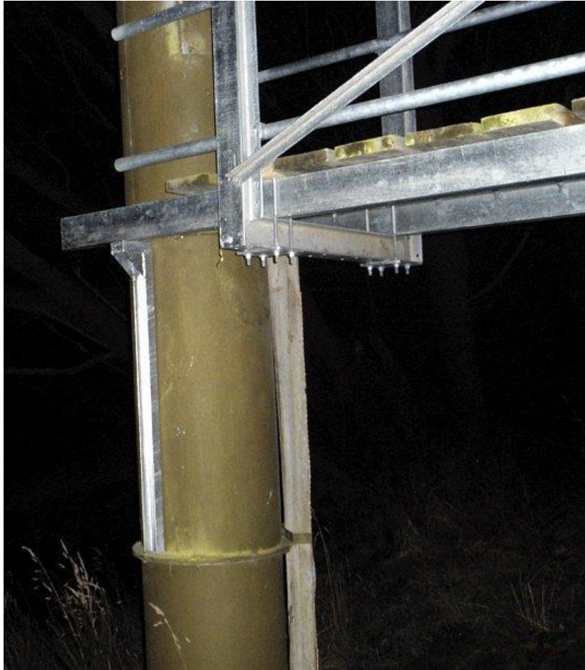
Figure 7 – Attachment to 600-mm stilling well with the new seat design (NIWA)
